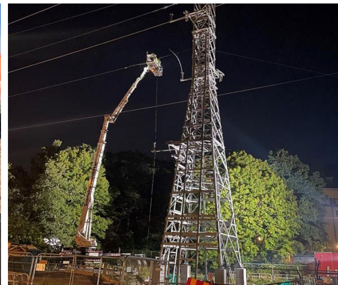
Stockholm's electricity grid was reinforced through new underground cables connected to an existing overhead line in the Royal National City Park.
