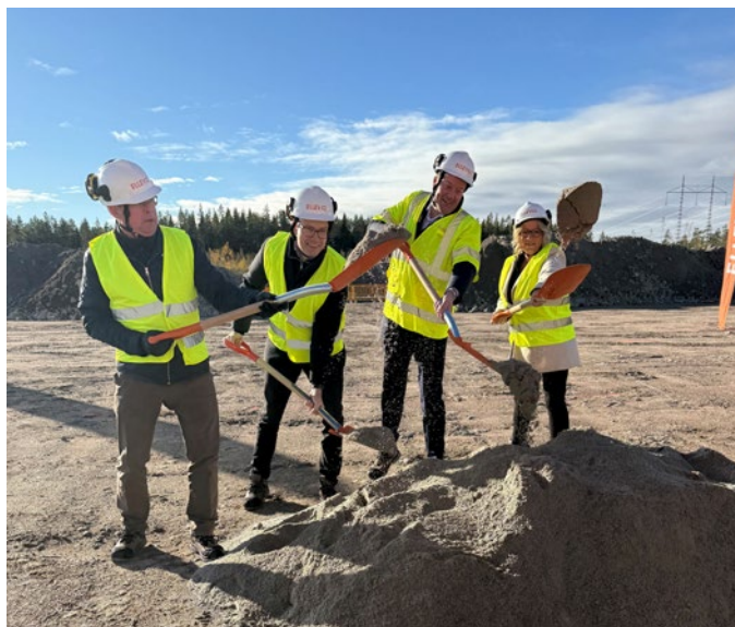
The construction of a substation in Njutånger in Hälsingland, began in 2025 with a groundbreaking ceremony attended by Ellevio's CEO Johan Lindehag (third from the left).
