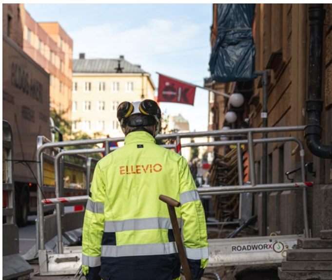
Replacement of grids that had reached the end of their technical lifespan was carried out at several locations in Stockholm's inner city.
